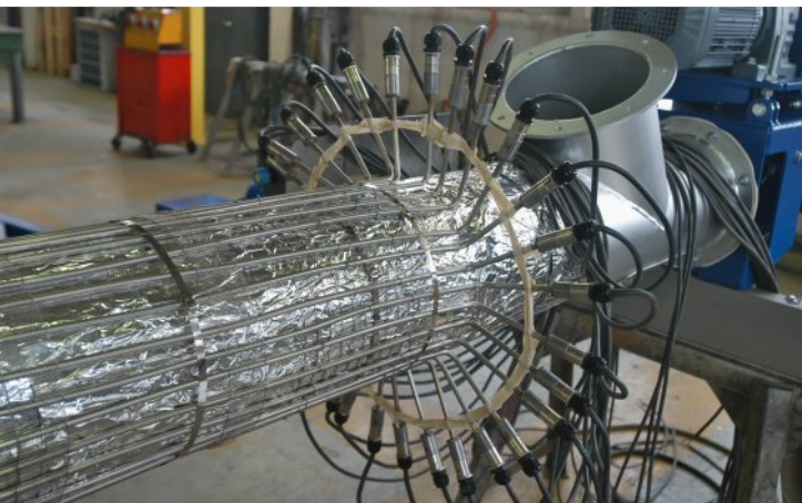
Workshop mounting of an electrical trace heating
