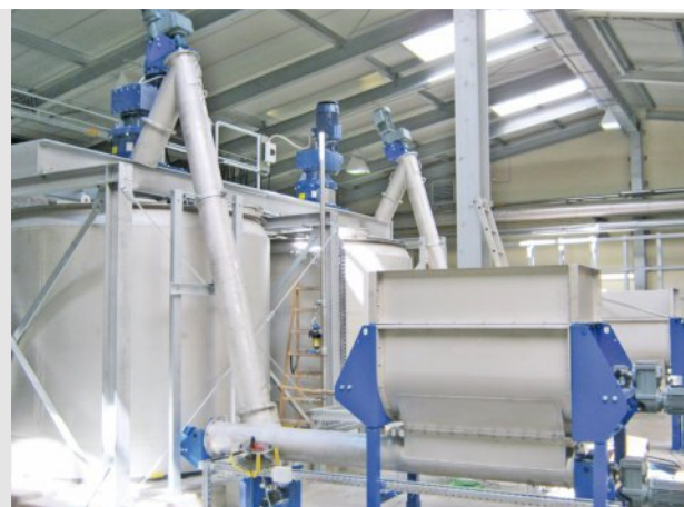
Pipe screw conveyor filling mixing vessels
