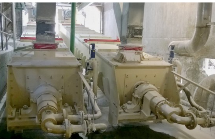
Screw conveyors in operation
