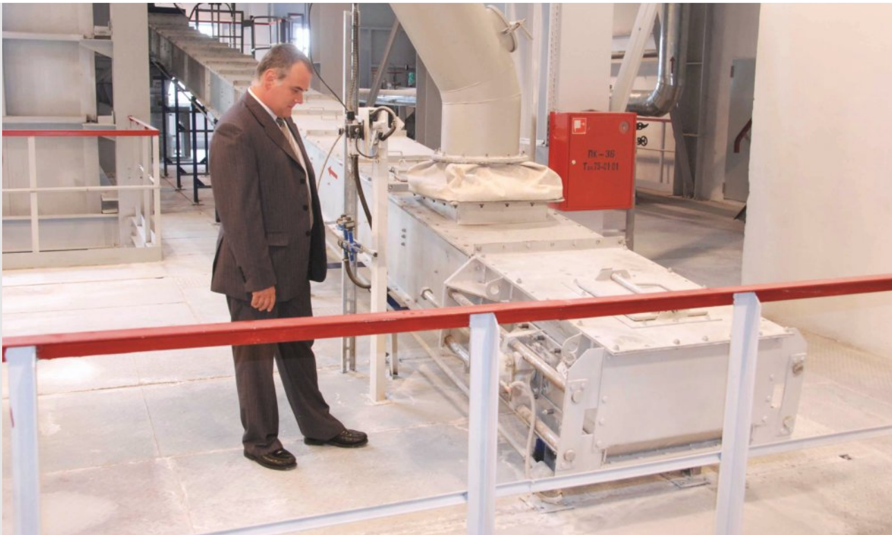
Trough chain conveyor for heavy sodium carbonate
