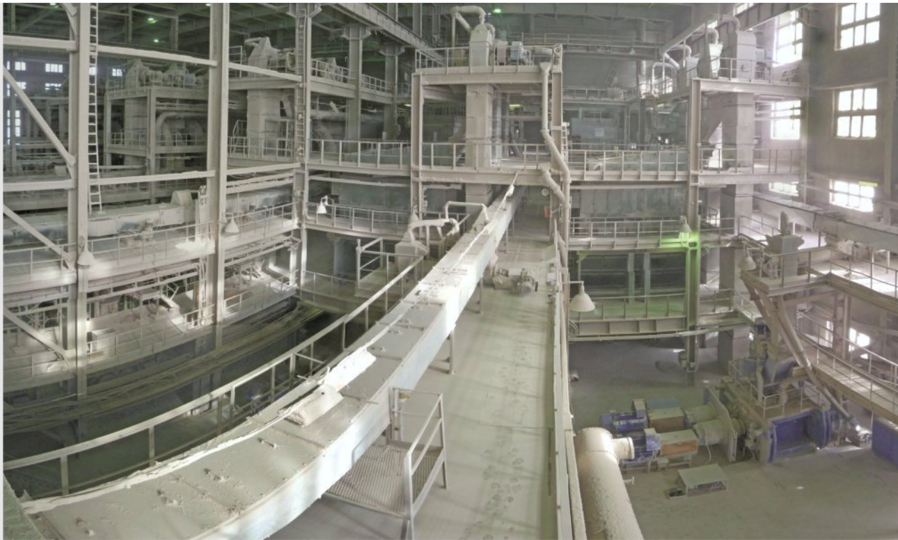
Potash transport for press loading; conveyor performance approx. 150 t/h
