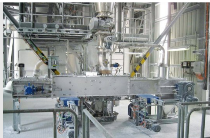
Distribution conveyor for sodium bicarbonate
