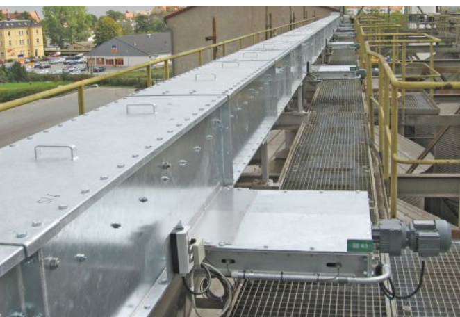
Oil seed conveying and distribution to silos
