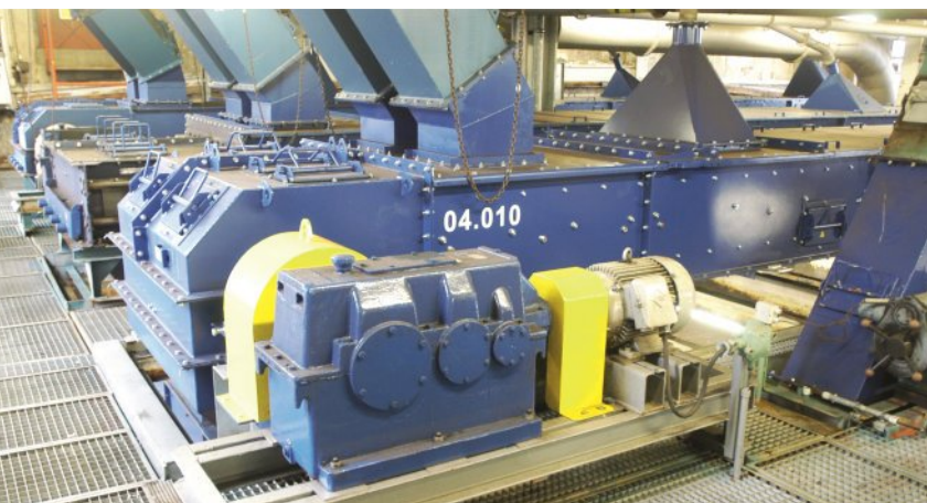
Trough chain conveyor drive station
